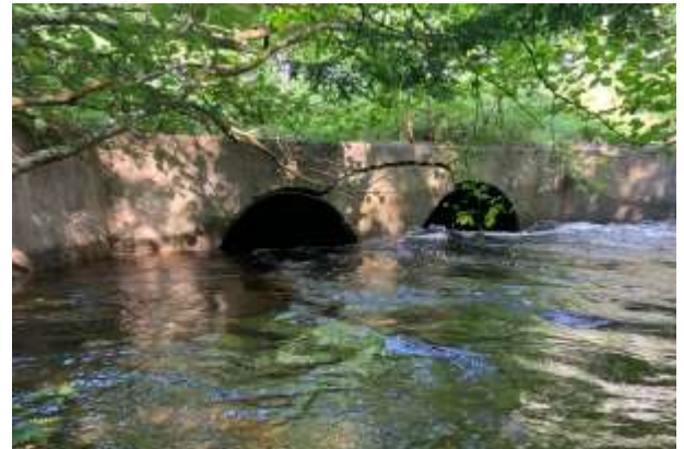
A double culvert with some clogged fencing.
